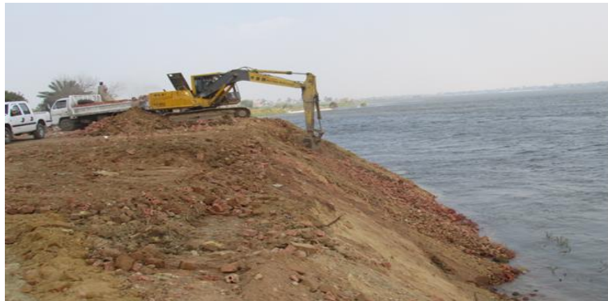
Photo (1): Removal of encroachment in BeniSeuif Governorate
