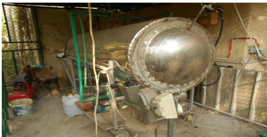
Figure (1): General view of digester and its attachments
